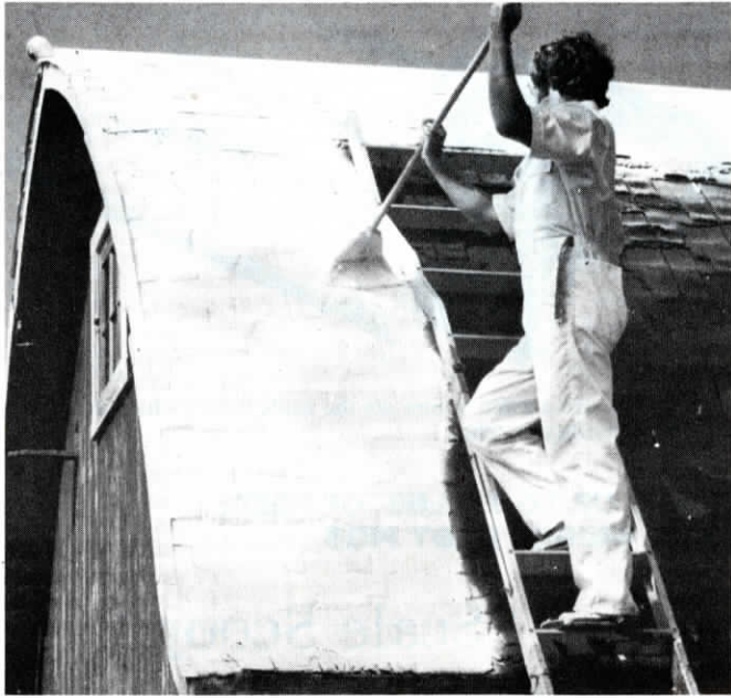
Rapid Roof was applied directly over the existing, badly-worn asphalt shingles on this barn roof.
