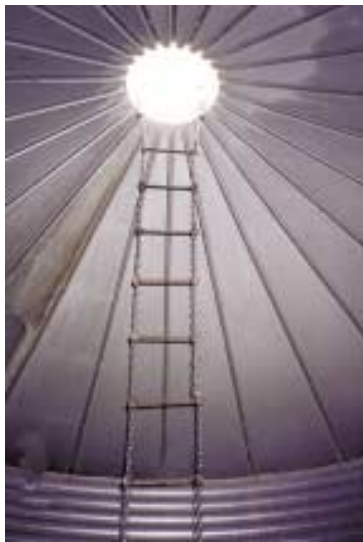
A pair of steel hooks at the upper end of ladder hang from bin's top porthole.
