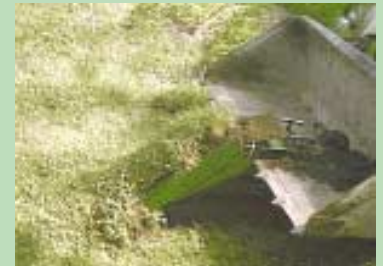
Unit guides soil up into the bucket where it can be piled or dumped.
