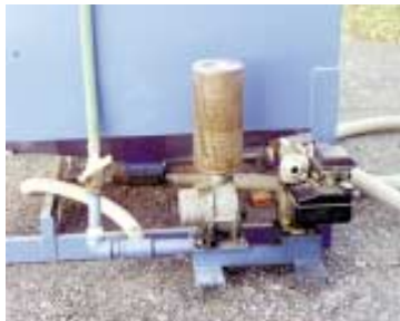
Blower is powered by a 5 hp horizontal shaft gas engine.
