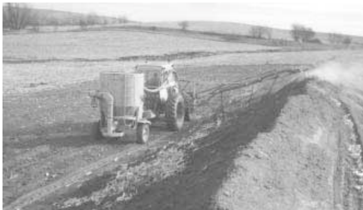
Seed is blown onto side of terrace. Chains that hang from boom cover it with soil.
