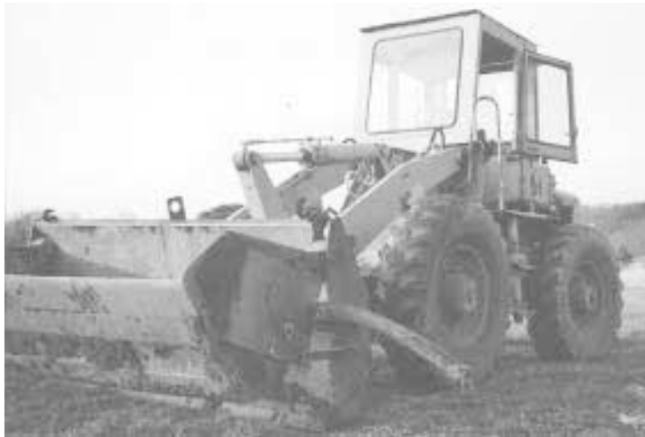
In order to cut through 3-in. dia. phone cable, Walter and Philip Miller added a 2-ft. sq. steel shear plate to the bucket of their IH payloader.
