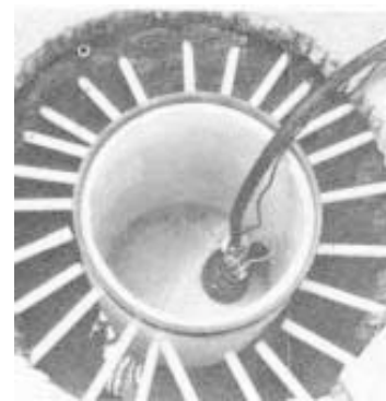
Drain pipes connect to a 50-gal. sump which is emptied by a pump.
