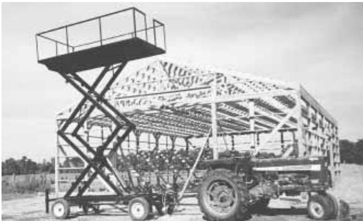
The 12-ft. long scissor arms for the lift are built from 2 by 6 rectangular 7-ga. tubing.
