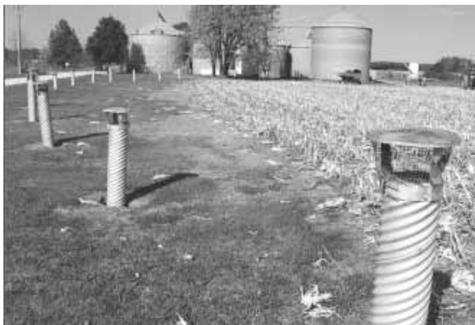
Ventilation system consists of 14 pipes buried 10 ft. deep. The pipes run 150 ft. from the barn to these stand pipes, which extend about 5 ft. above ground.
