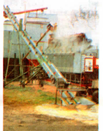
Augers load grain into "cross auger" that distributes grain to holding bins.
